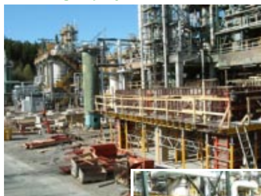
Extensive building work is in progress at the unit in Stenungsund to prepare for the transition to natural gas as a replacement for fuel oil.
