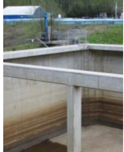
Equalization tank 2 at the wastewater treatment plant in Perstorp, Sweden.
