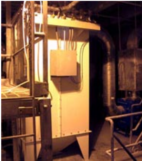
The unit in Florence, USA, has implemented a dust capture project reducing airborne dust and eliminating some materials handling.
