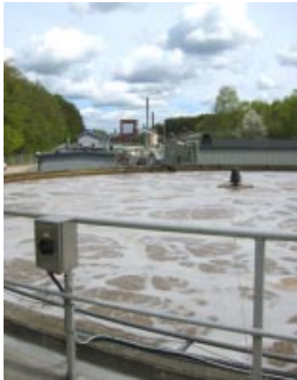
Aeration tank 2 at the wastewater treatment plant in Perstorp.
