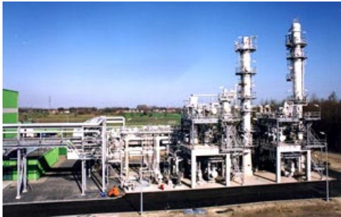
Distillation plant NX 795 and BEPD.
