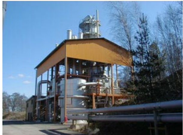
Formalin plant 5 at the Perstorp site.
