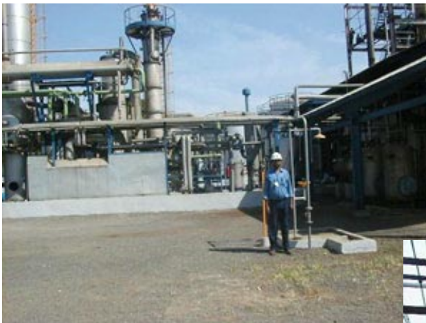
In front of the formalin plant after implemented measures: An emergency shower has been installed. Personnel have a uniform, protective shoes and a helmet.
