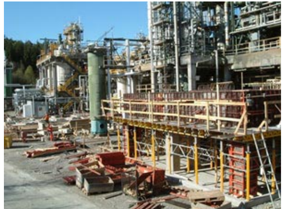
Extensive construction work is in progress at the unit in Stenungsund, Sweden, to replace heating oil with natural gas.
