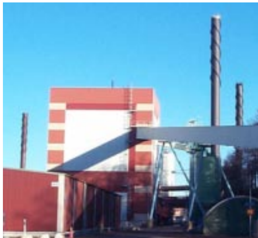
The steam power plant of Perstorp Support AB is located in the Perstorp Industrial Park, at the largest unit of the Group. The switch from coal to biofuel (mainly wood chips) took place in 1991. The main fuels are wood chips, returned wood and peat.
