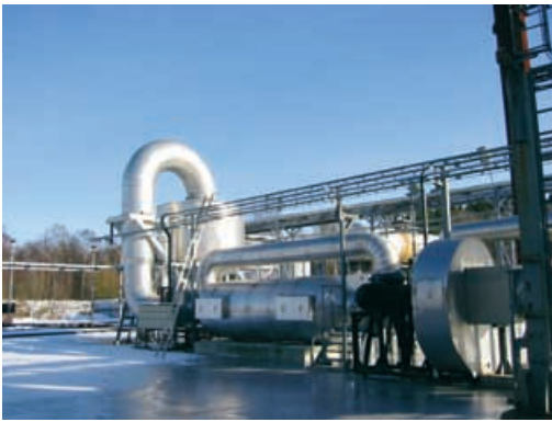
There are 15 catalytic incineration facilities at different production plants at the site in Perstorp, Sweden. The largest facility comprises three lines - each with a capacity of 25 000 Nm 3 /hour.
