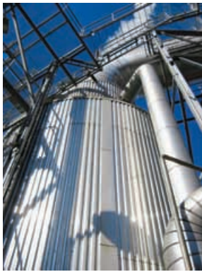
The flue gas scrubber at the steam power plant.
